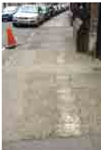
Poor pavement outside St George's, Castle Street
