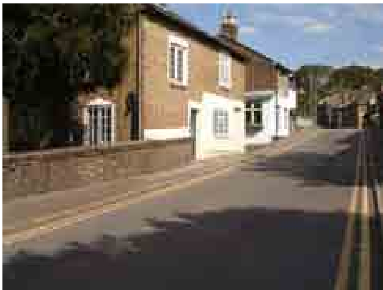
Brick footings of a road bridge crossing the River Bulbourne next to 25 Ravens Lane
