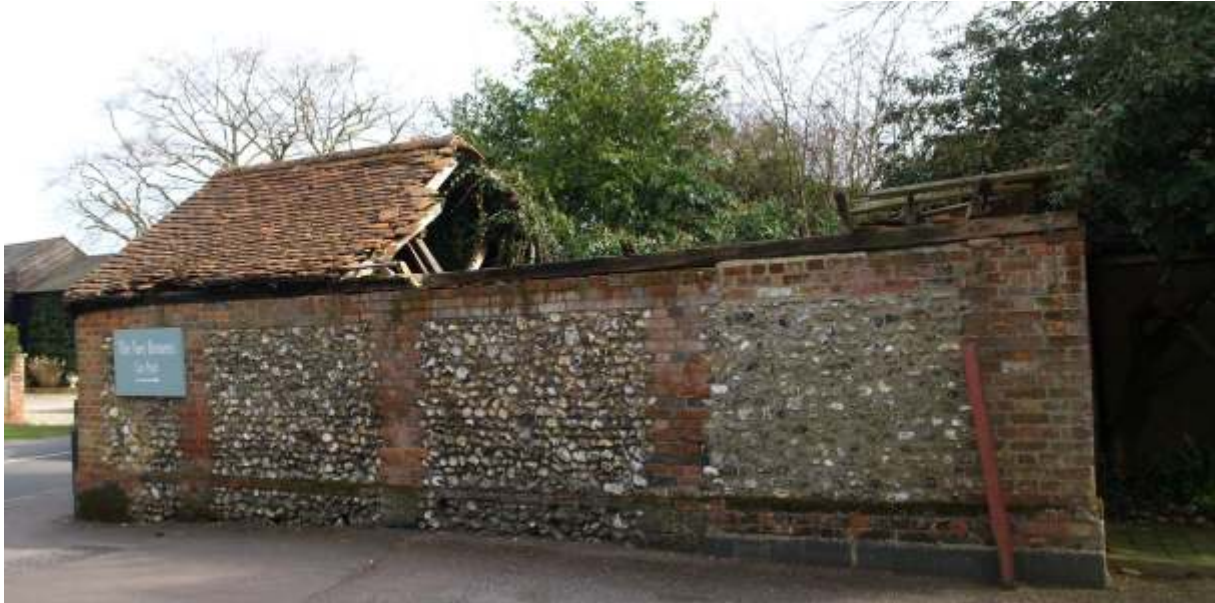
Collapsing outbuilding to rear of Two Brewers
