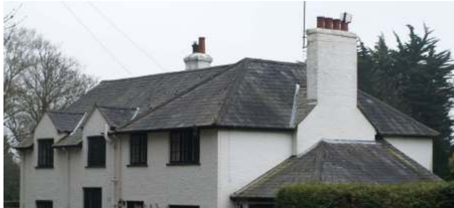
Slate was used from c.1800 in Chipperfield. Pitches tend to be flatter.
