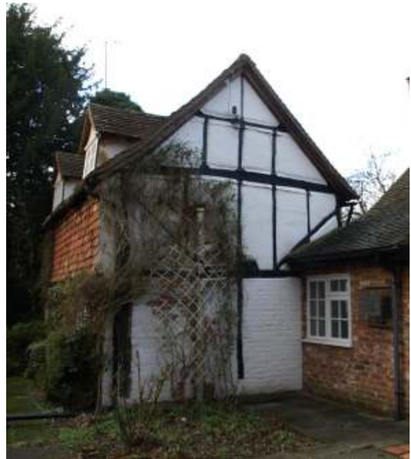
Groves Orchard: the tile-hanging to the frontage conceals a C17th timber-framed building
