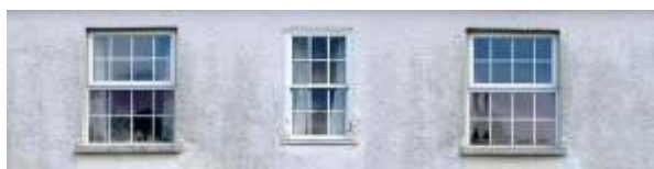
Inappropriate replacement windows here upset the rhythm of the fenestration of this house
