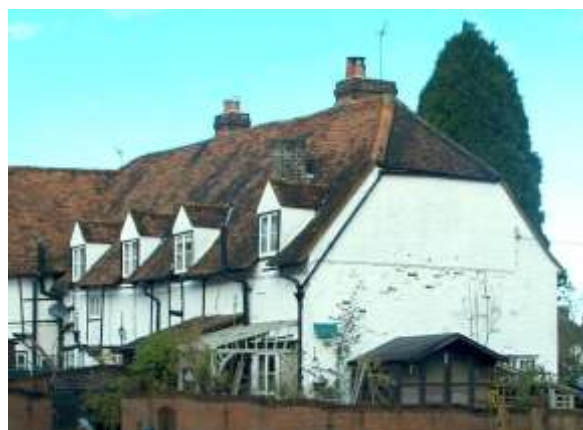
Satellite dishes, poor quality lean-tos and sheds, lack of maintenance
