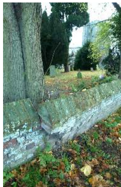
Damaged churchyard wall
