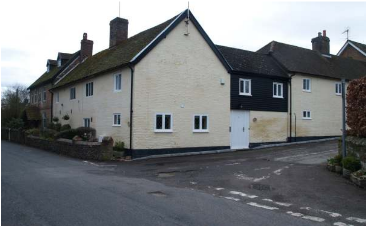
Poor road surfacing at junction with Roman Road
