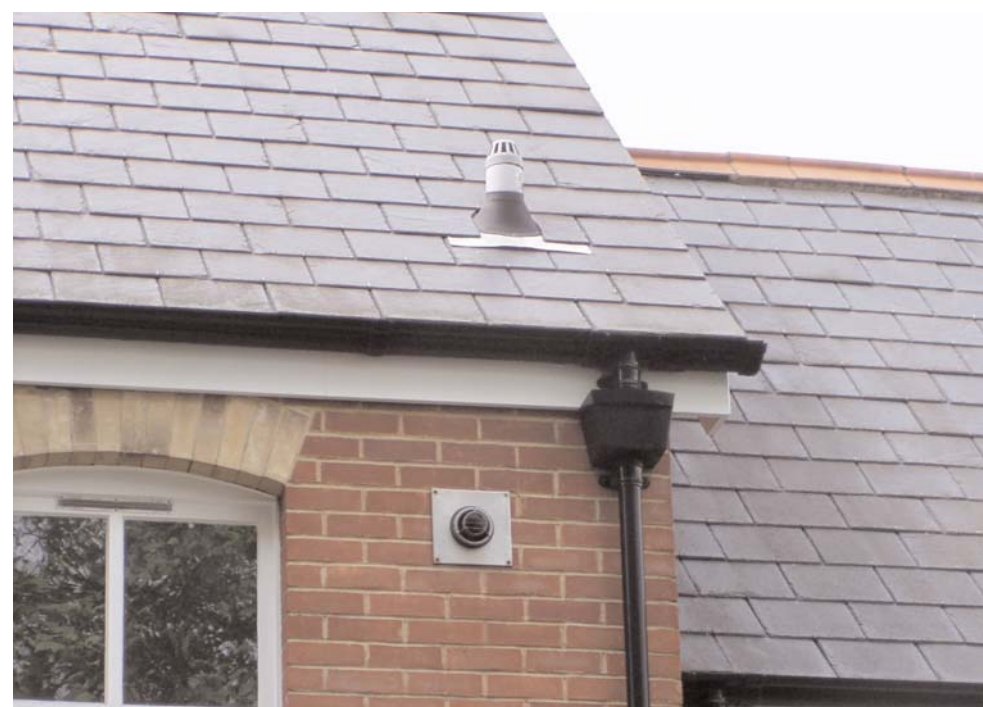
The roof on this house demonstrates a common slate roof. Artificial slate made of cement is used frequently with little noticeable difference.
