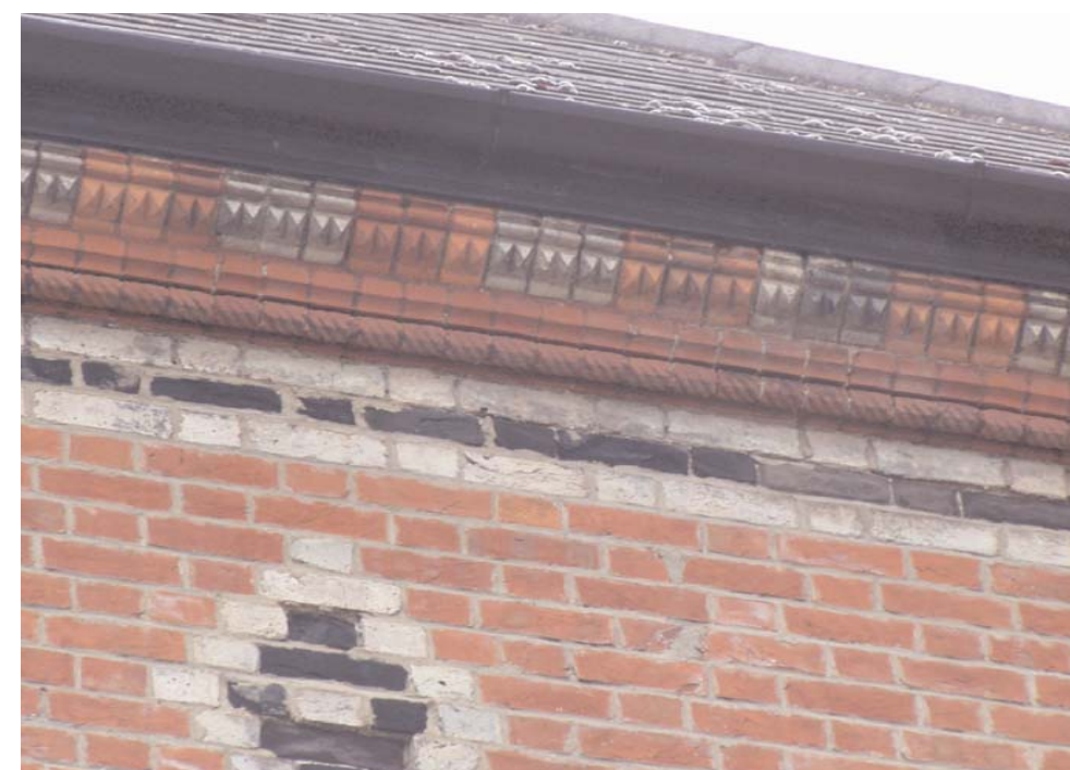
The Victorian decorative brickwork contains blue bricks that have been fired longer in their kilns.
