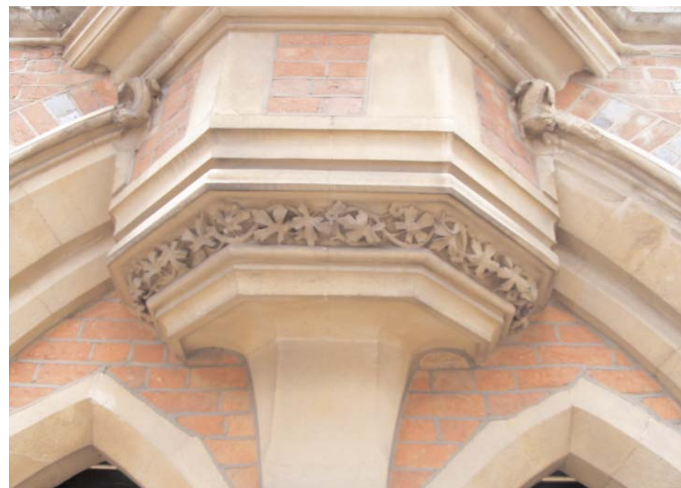
The keystone of the Town Hall arched entryways are made with brick and decorative limestone.
