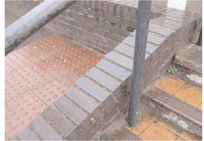
The area around the steps leading from the street to the upper level of pavement on the west side of the High Street displays a discordant mix of materials, including tiles, ridged tiles, machine-made bricks, older brickwork, non-slip pavers, and concrete blocks all within a few square metres.
