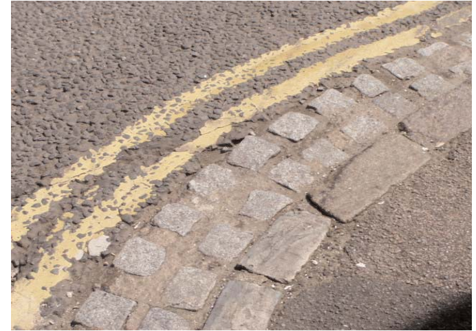
The durability of granite has made it the preferred material for kerbs and gullies.
