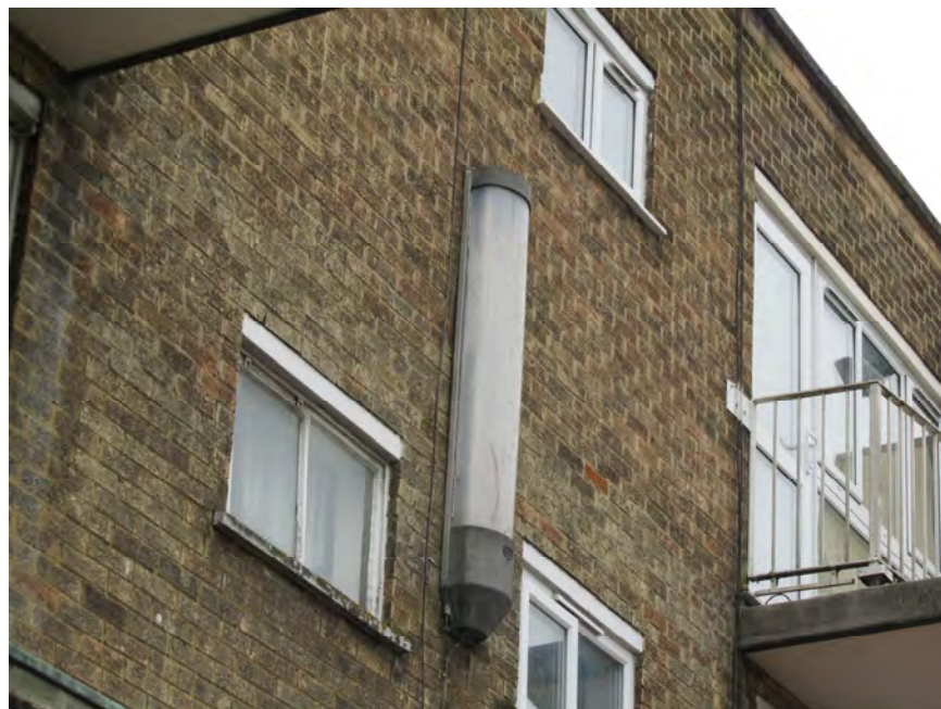
Marlowes west side: Original wall mounted lamp. There are a few remaining along this frontage.
