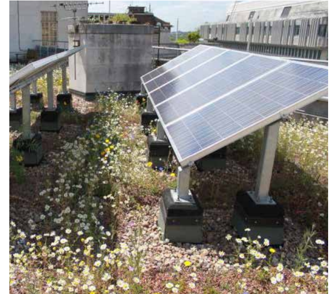
Renewable PV Panels and biodiverse green roof
