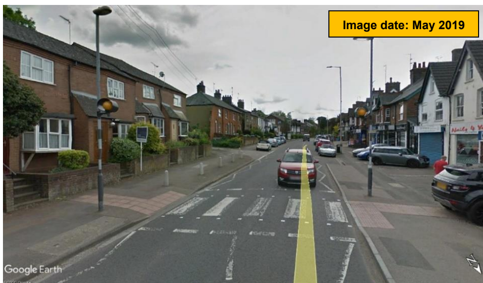
Figure 5-18: Faded markings on zebra crossing on the B4635 (Western Road/Aylesbury Road)
