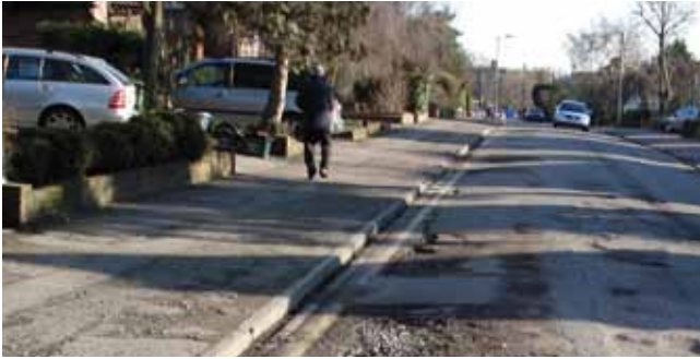
Maintenance of the road system is presently considered the highest priority by the public
