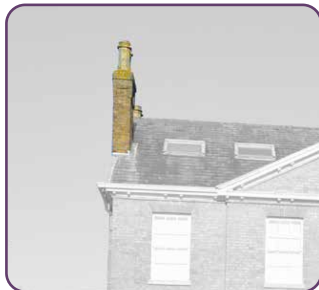
Figure 73: Chimney stack with yellow brick and the sunlight dormer in the Village Centre.
