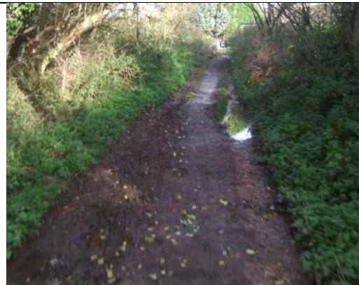
Figure 6 – Surface condition on Marshcroft Lane
