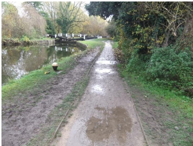
Figure 1 – Poor Towpath condition in Berkhamsted
